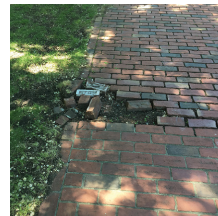
broken brick paving
