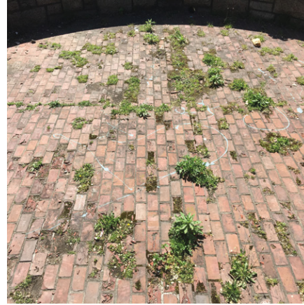
broken brick paving
