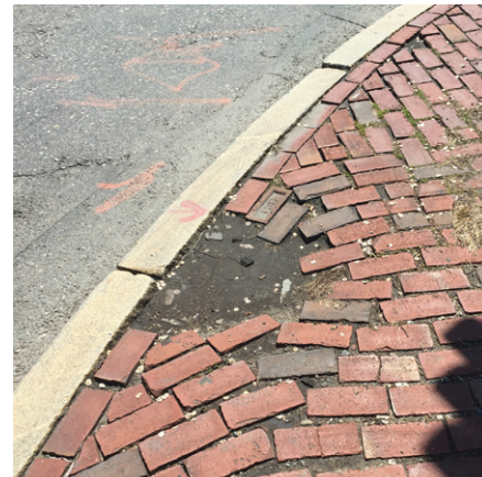
broken brick paving
